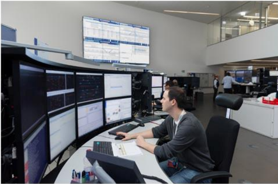
Control room with WinCC OA
